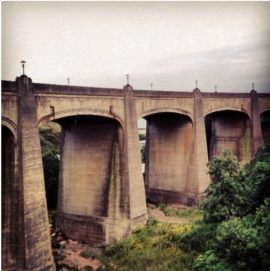
The Jubilee Bridge, opened in 1935, is struggling to cope with the weight and amount of current traffic.
